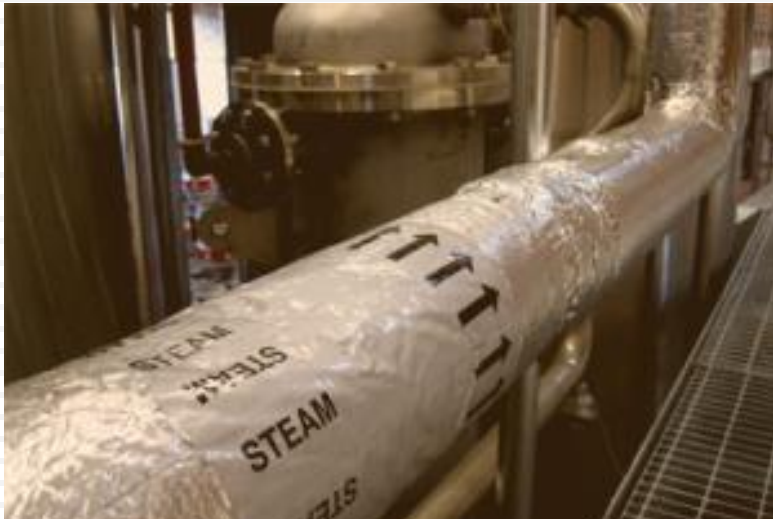
Proper Insulation at Steam Lines
