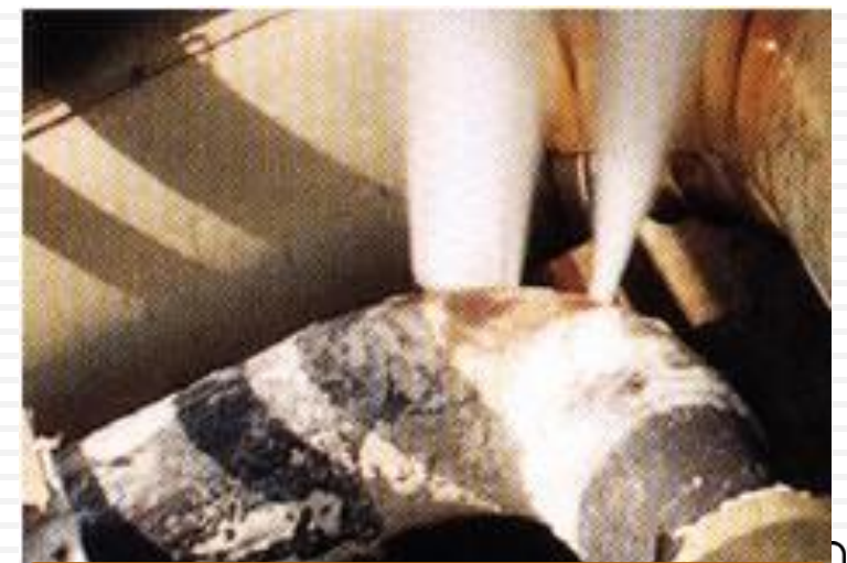
Through material deterioration
