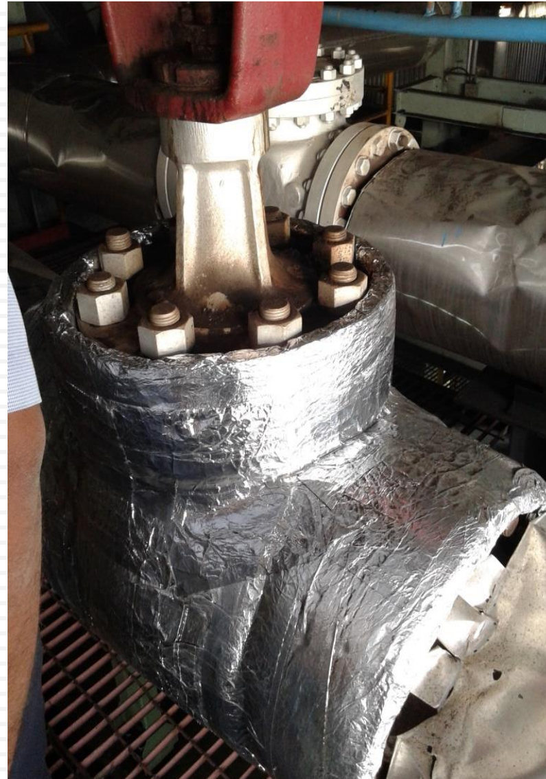
Proper Insulation at Valves
