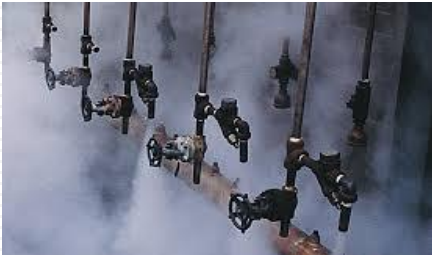
Through Faulty Traps
