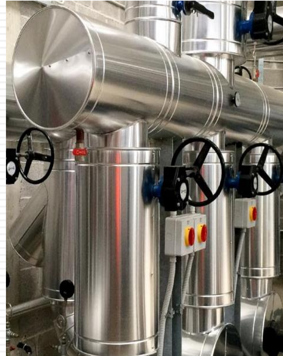
Proper Insulation at Steam Distribution
